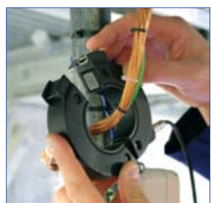
PD activity in cables is monitored using Radio Frequency Current Transformer (RFCT)
