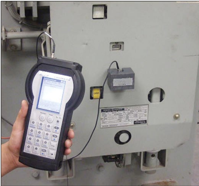
Figure 4 —A vibration sensor is attached to a breaker in order to obtain critical operating characteristics.
