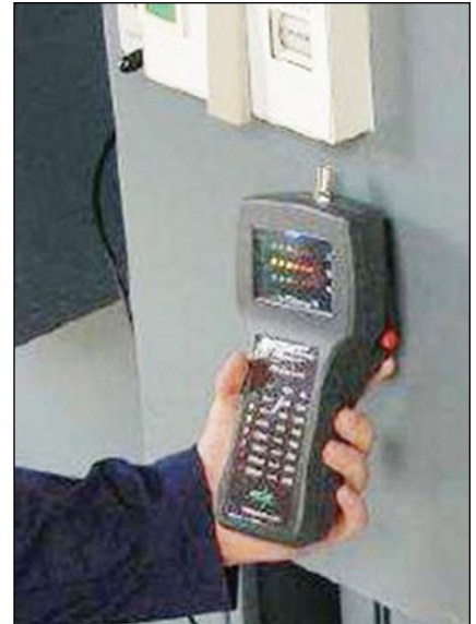
Figure 3 — Using a simple hand-held partial discharge detector to ensure no electromagnetic signals indicative of insulation failure are occurring within the switchgear enclosure, a wise safety check
